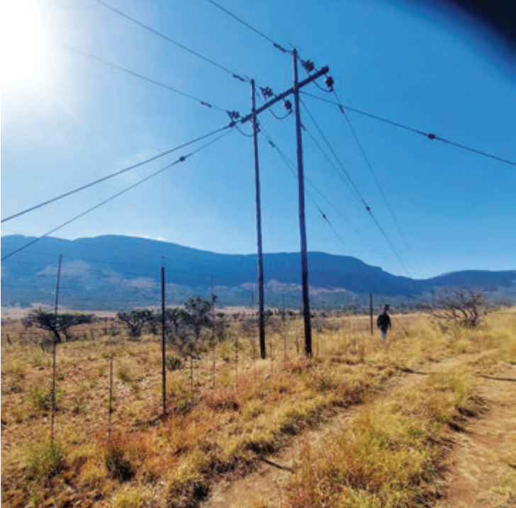
A closer look at the Eskom wishbone-style powerline structures near Marakele, where recent vulture deaths occurred.
